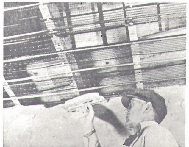
Fig. 5—Application of Plaster to Lath and Tubes Tubes attached to joists. Lath below tubes, also attached to joists. First coat of plaster applied to lath and tubes.
