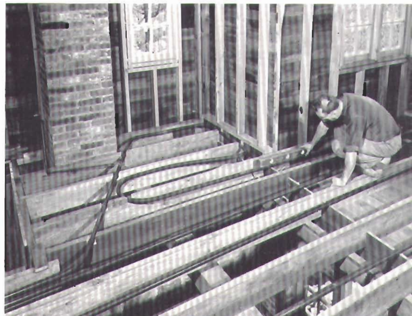
Rayduct floor piping in the second story of a dwelling at Lancaster, Pa.
