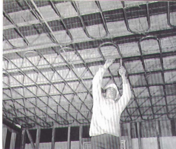
Right: Rayduet ceiling coils in place in the home shown at left.
