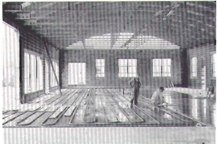
In building shown at top of page, Rayduct rests on 4-in. slab over 7-in. stone fill, and is covered with a 3-in. slab of concrete.
